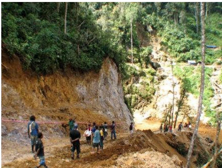
Road cut across spur with part of artisanal mining area in background.
